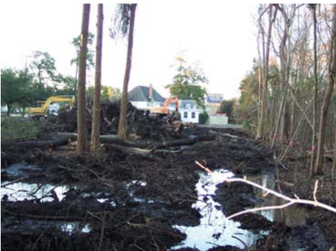
Pawleys Island isolated wetland being cleared and filled under nationwide permit with no prior public notice.
